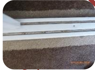
Requires to be cleaned
