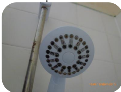
Requires to be cleaned
