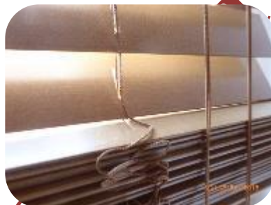
Requires to be cleaned
