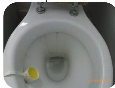
Requires to be cleaned
