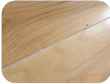
Requires to be cleaned
