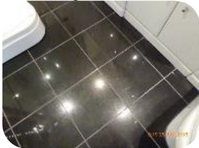
Requires to be cleaned
