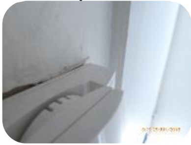
Requires to be cleaned
