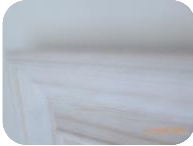
Requires to be cleaned
