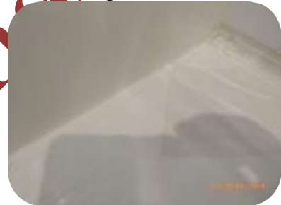
Requires to be cleaned
