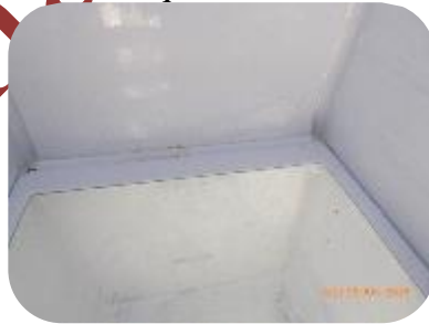
Requires to be cleaned
