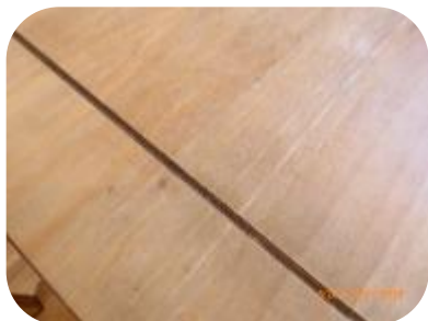
Requires to be cleaned
